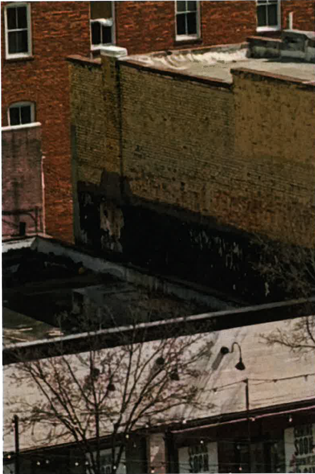
Photo 9: 205 S. Wilmington Raleigh, NC (03/19/2026) : Parapet of 205 shows independent from 209 S Wilmington
