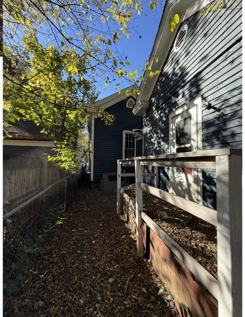
Side Porch/Deck to be Rebuilt
