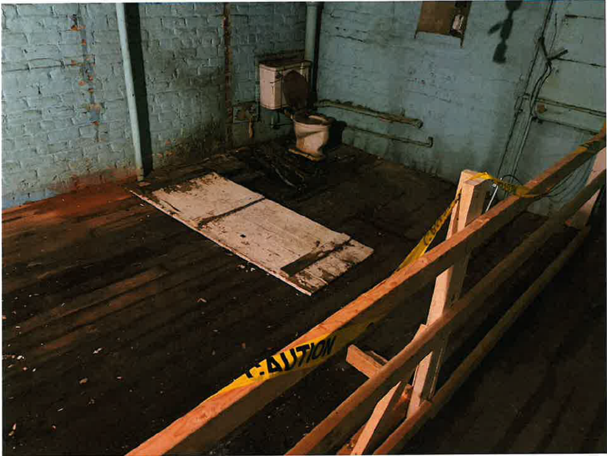
Photo 17: 209 S Wilmington St Raleigh, NC (03/19/2026) : 3 rd floor rear major structural damage from plumbing and roof leaks.
