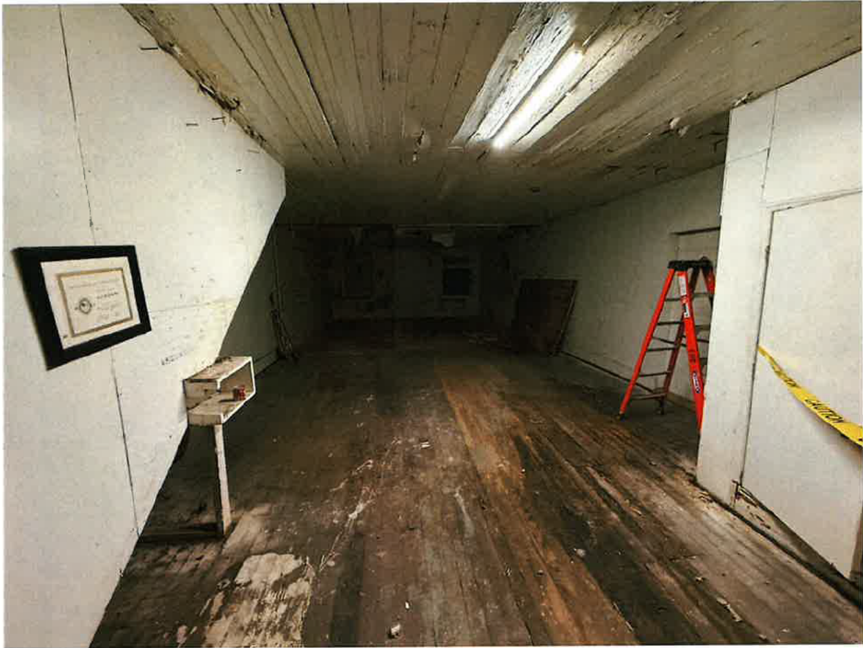
Photo 9: 209 S Wilmington Raleigh, NC (03/19/2026) 2 nd floor Interior Facing West (Wilmington St) Wood flooring has been patched several times and is rotting. Same for T&G ceiling.
