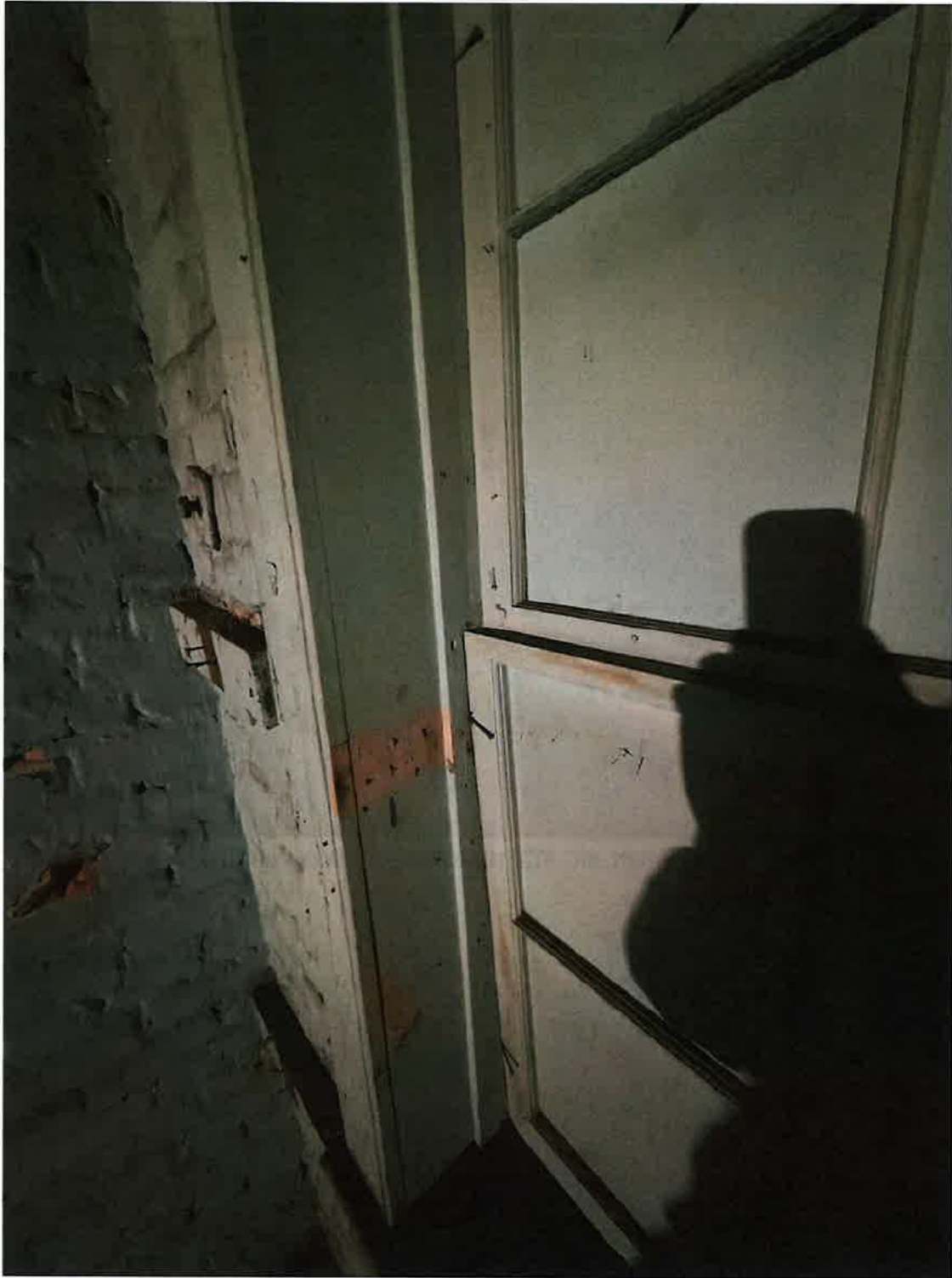
Photo 18: 209 S Wilmington St Raleigh, NC (03/19/2026) 3 rd floor front, window sashes, tacked in place, Portland based stucco and wire lath beneath. Unknown if sashes are original.
