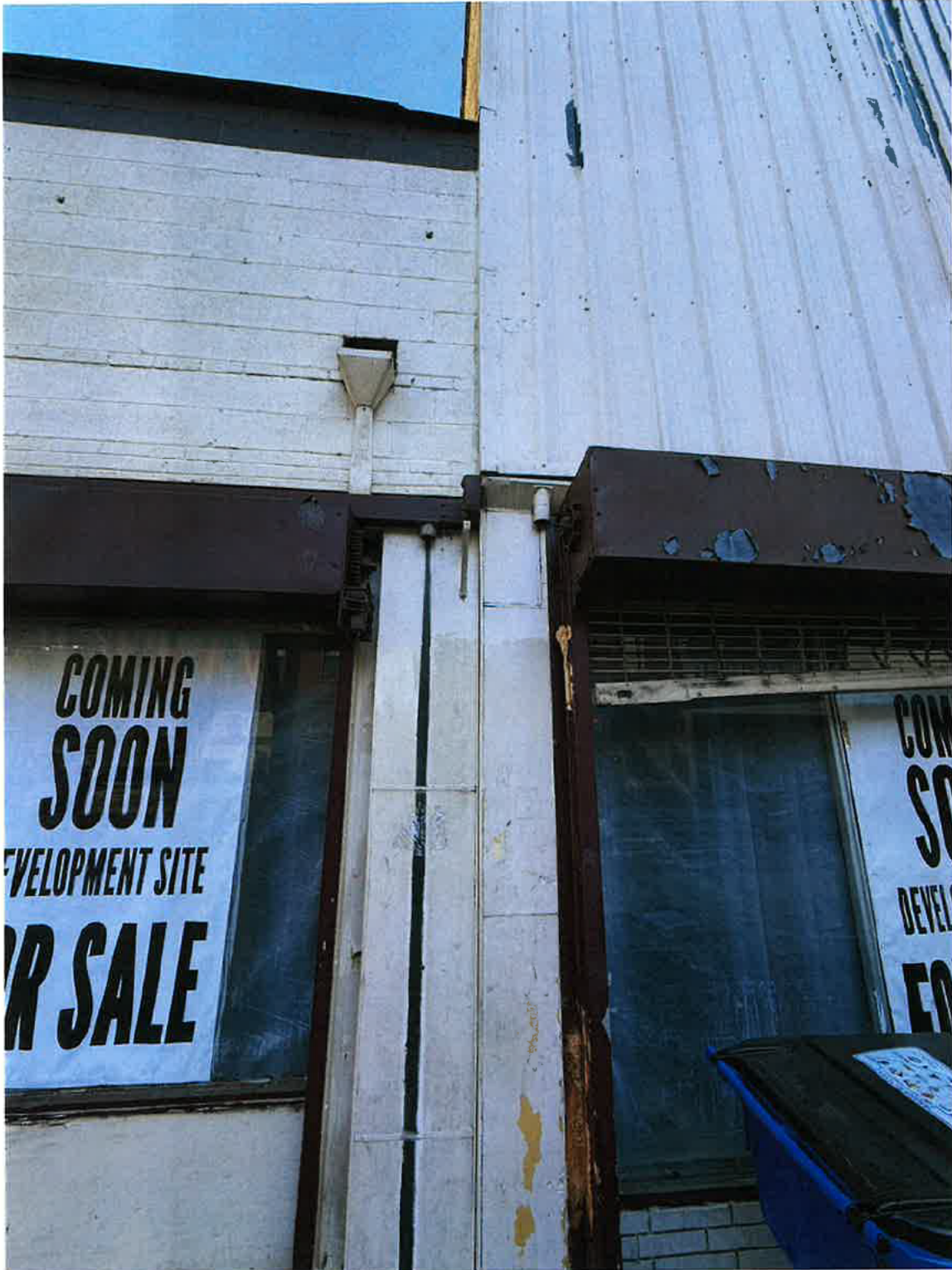
Photo 19: 209 S. Wilmington St Raleigh, NC (03/19/2026) 209 S. Wilmington St. independent of 205 S Wilmington St. The load bearing masonry wall is separate from 205, however, much of the north masonry wall was removed at the 1 st floor
