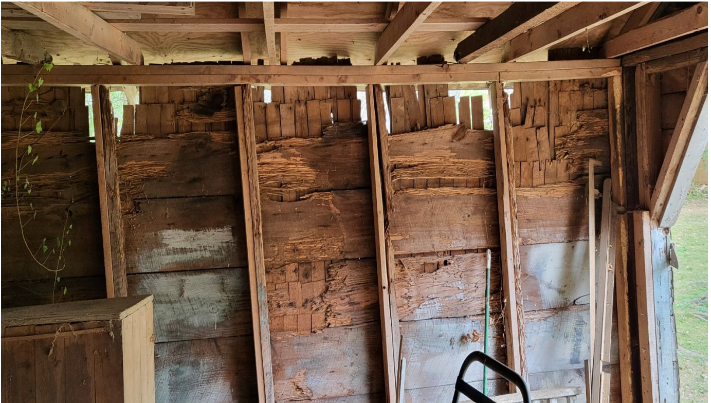
Inside West facing wall of garage, showing deterioration
