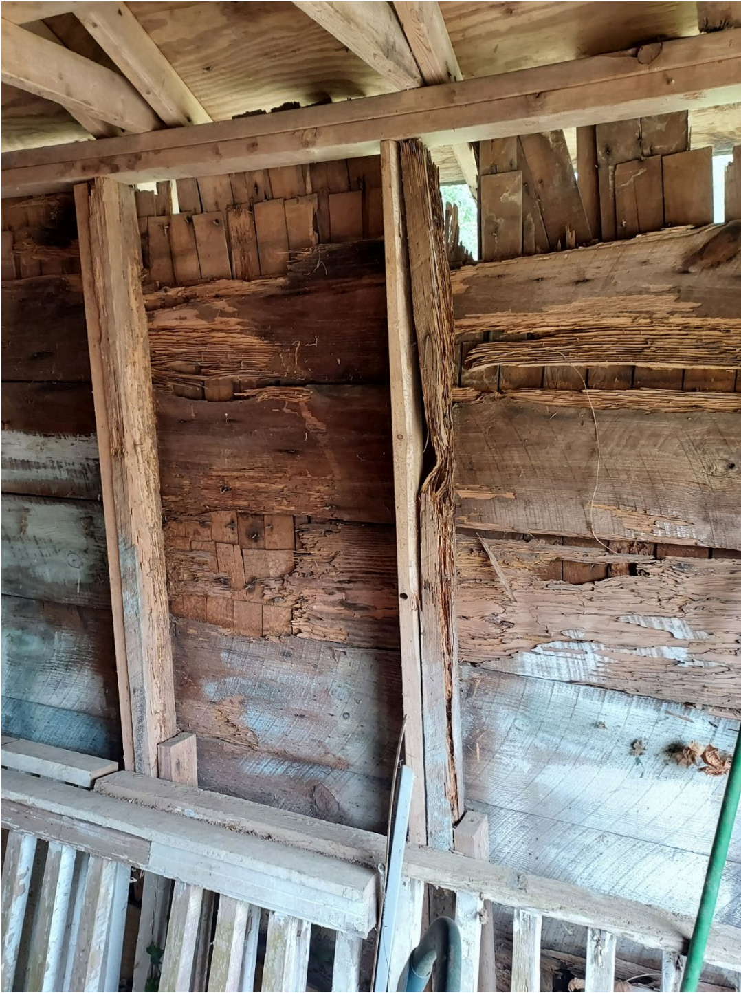
Closer view of inside West facing deteriorating wall and columns
