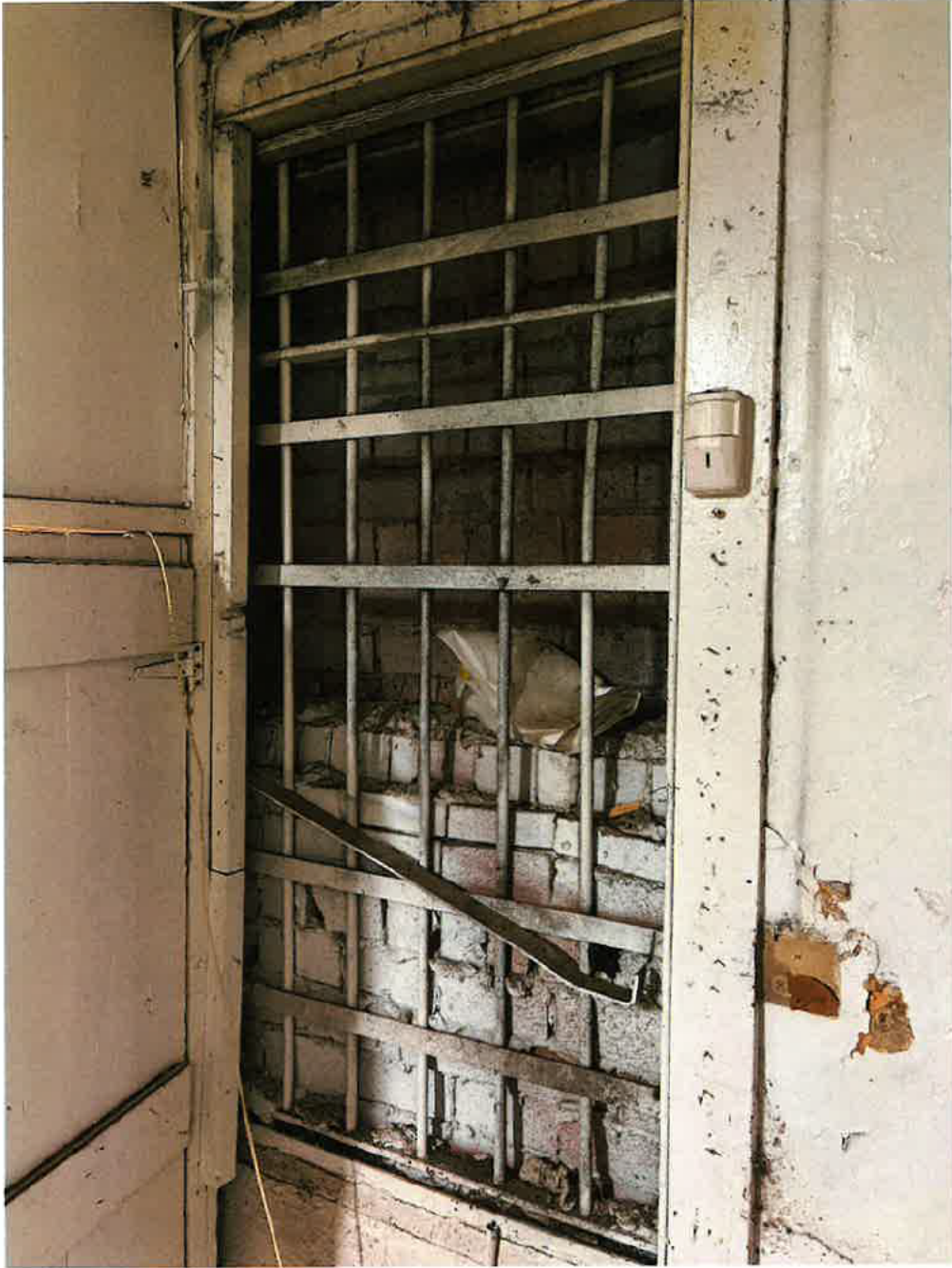
Photo 11: 209 S Wilmington Raleigh, NC (03/19/2026) 2 nd floor, rear bricked in window. All doorways and window openings on the rear façade are bricked up with little or no remaining millwork.
