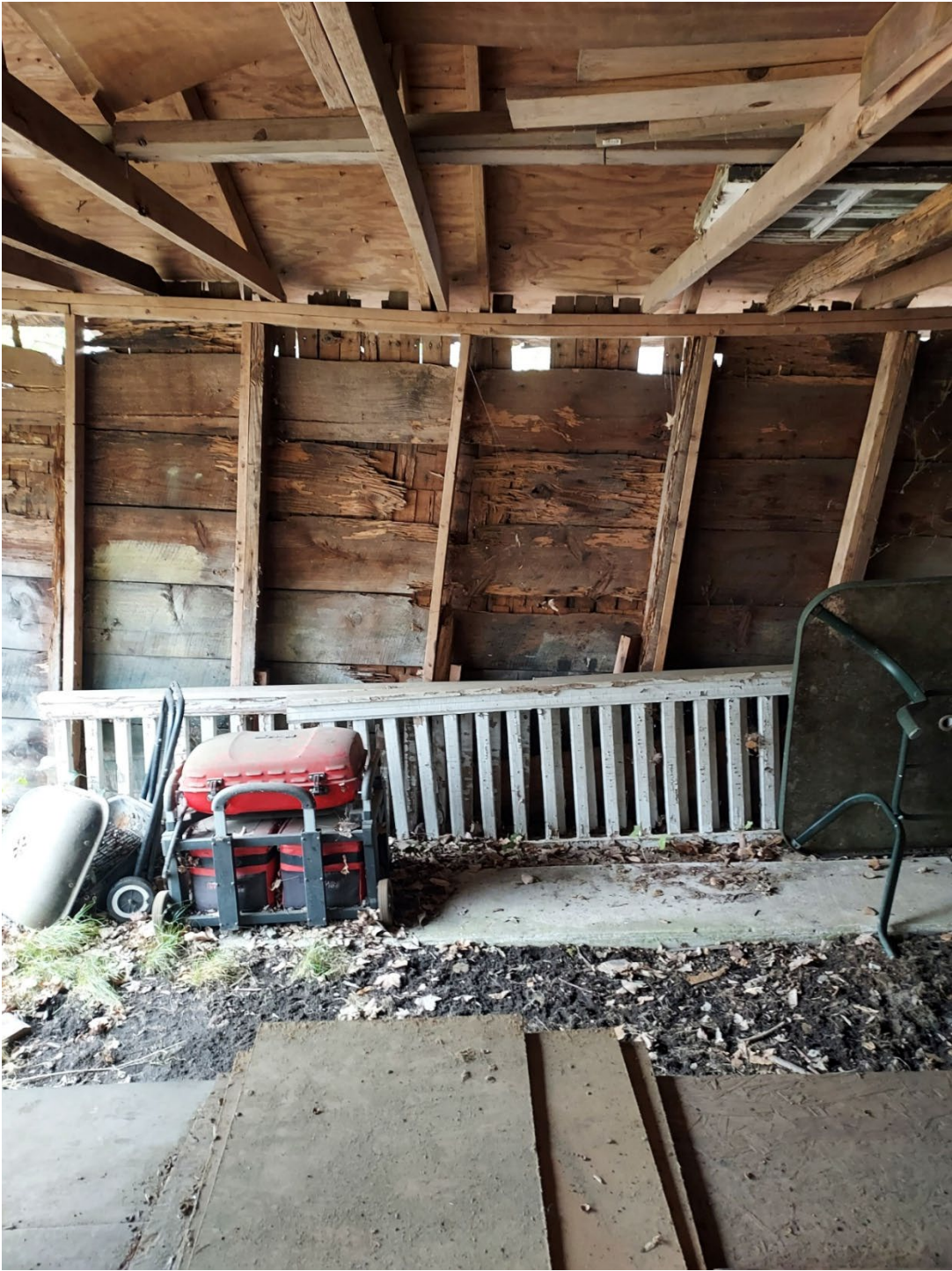
Inside East facing wall of garage, showing leaning 2"x4" columns
