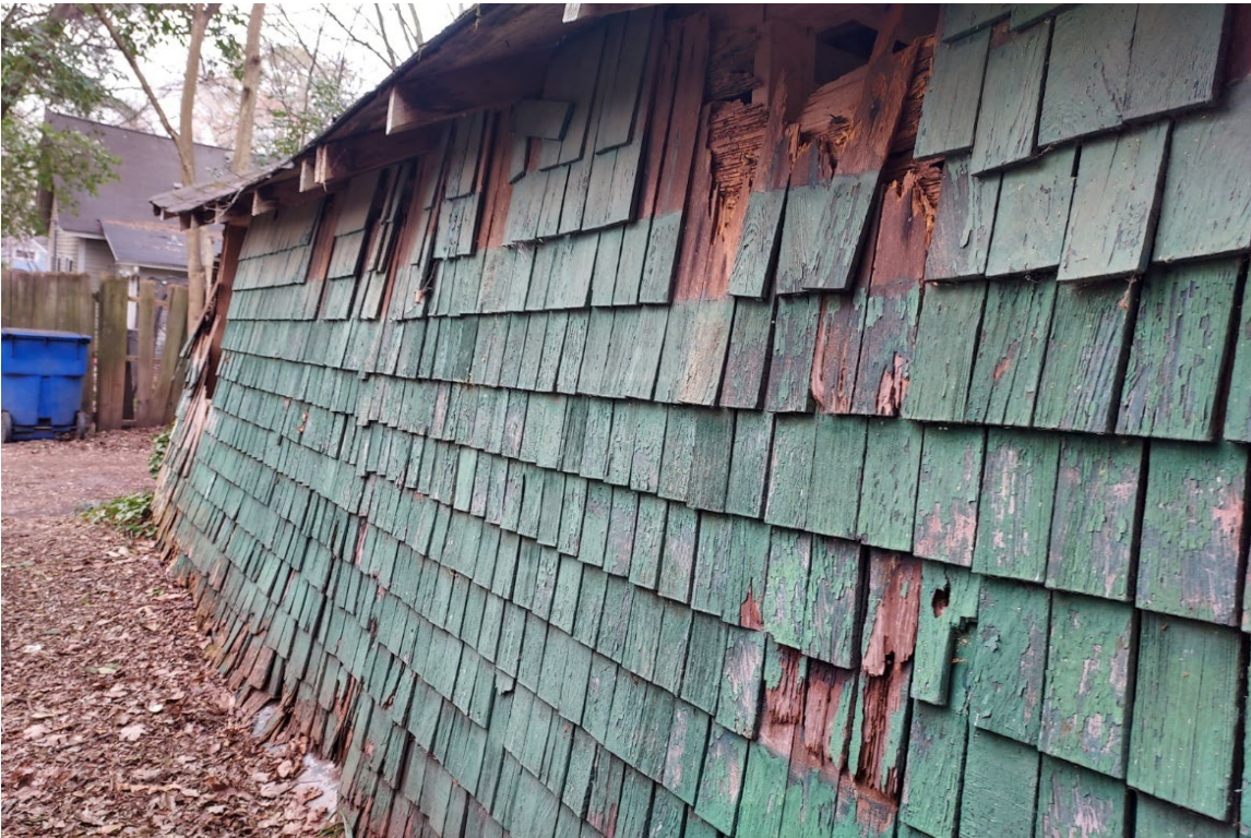
Damage to outside East wall from the front corner of the garage
