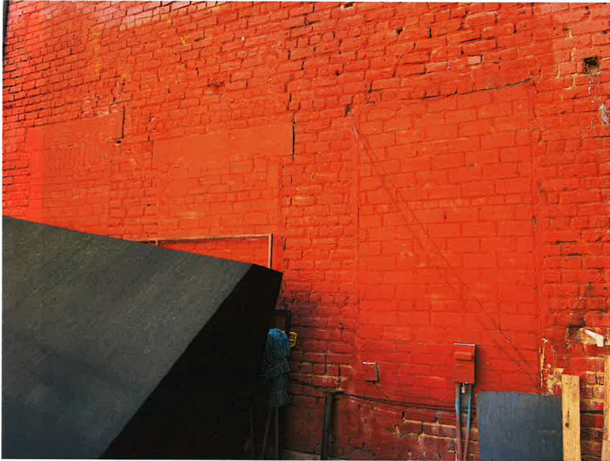
Photo 24: 209 S Wilmington St. Raleigh, NC (03/19/2026) Rear Façade, bricked in openings
