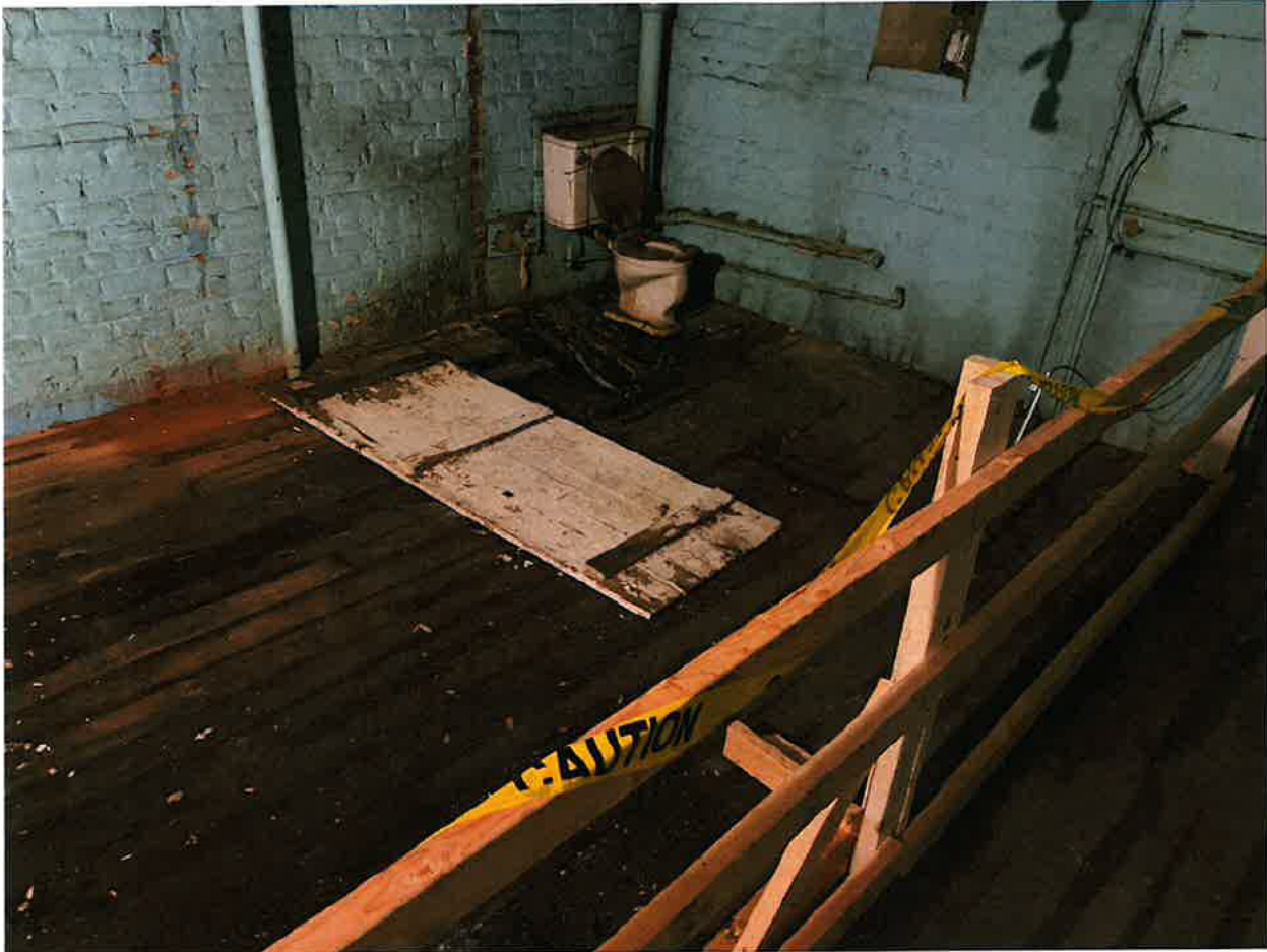
Photo 17: 209 S Wilmington St Raleigh, NC (03/19/2026) : 3 rd floor rear major structural damage from plumbing and roof leaks.
