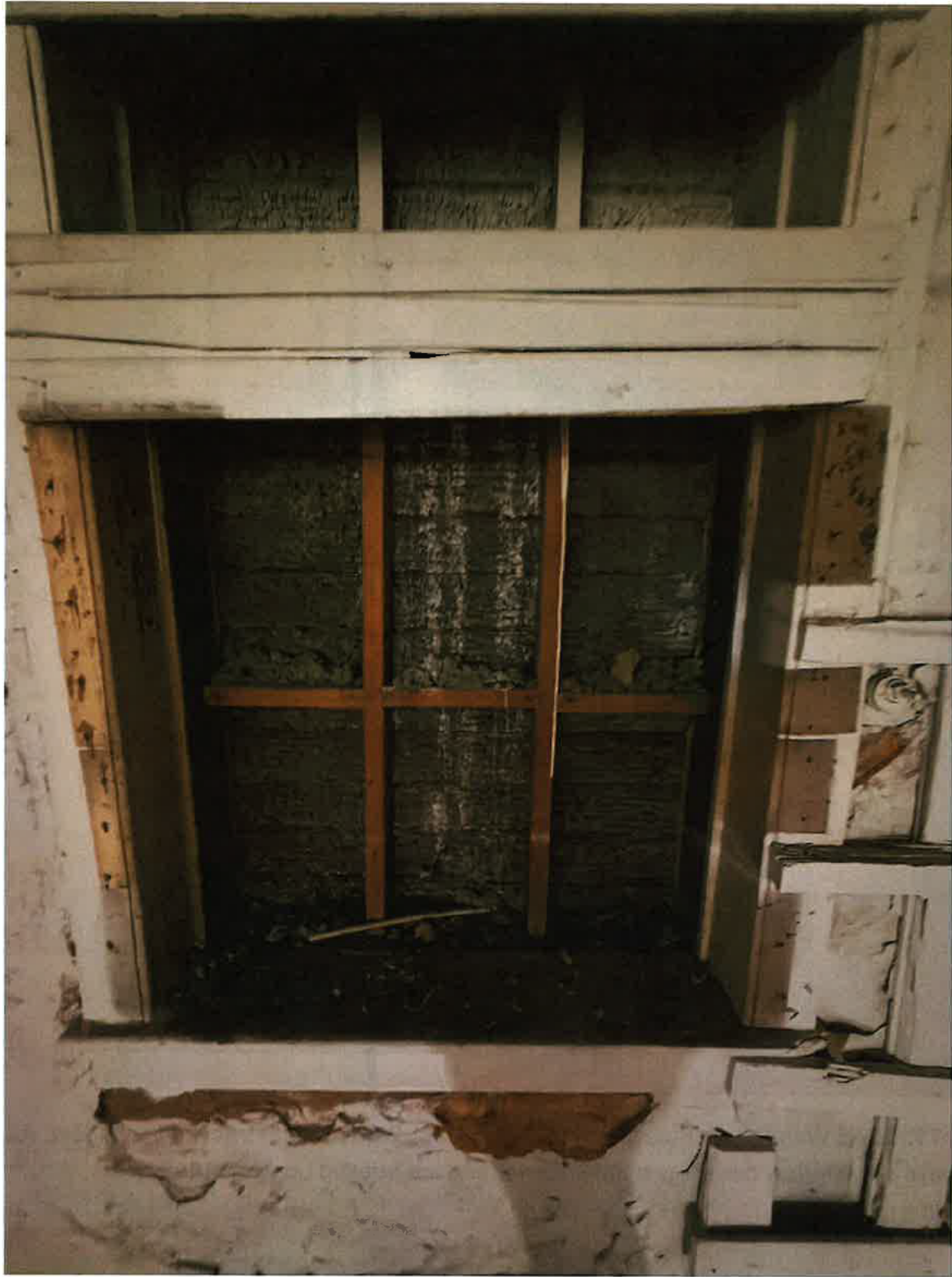
Photo 12: 209 S Wilmington Raleigh, NC (03/19/2026) 2 nd floor, front window opening with wire lath and Portland based stucco rendering directly to the masonry façade. No sashes and little or no original millwork.
