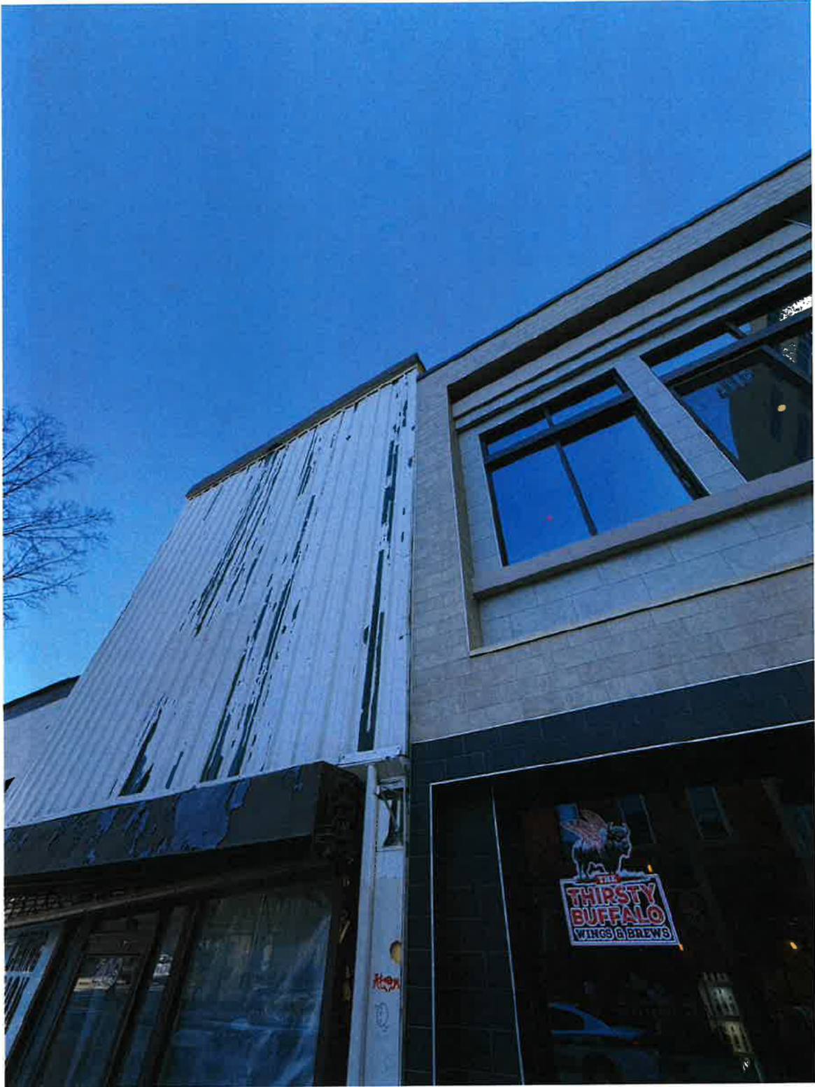
Photo 21: 209 S. Wilmington St Raleigh, NC (03/19/2026) 209 S. Wilmington St. and 211 S. Wilmington facades appear to be structural independent.
