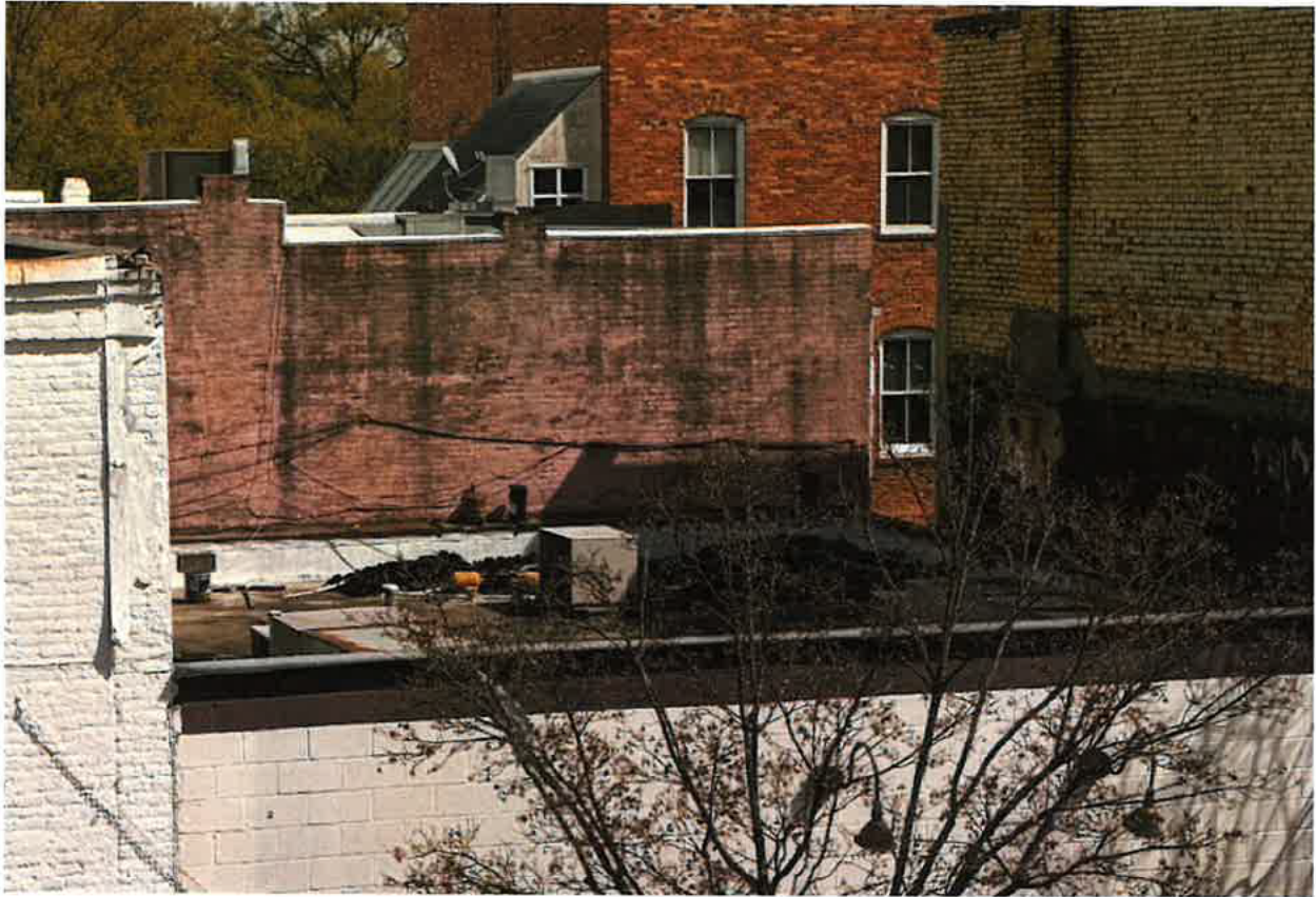
Photo 10: 205 S. Wilmington Raleigh, NC (03/19/2026) : Rear Parapet of 205 shows independent from 110 E Hargett St.
