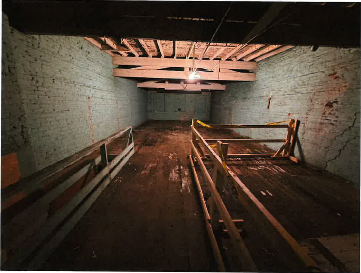
Photo 14: 209 S Wilmington Raleigh, NC (03/19/2026) 3 rd floor Interior Facing East (Wilmington St) Significant rot on hardwood flooring and severe damage to floor and roof structures as well large cracking on North and South masonry walls.
