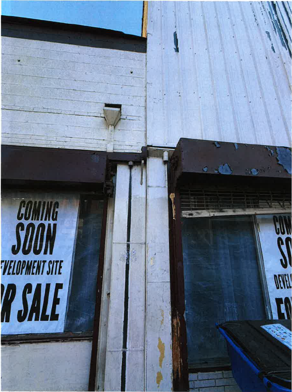
Photo 8: 205 S. Wilmington St Raleigh, NC (03/19/2026) 209 S. Wilmington structure and cladding appear to be independent of 205.
