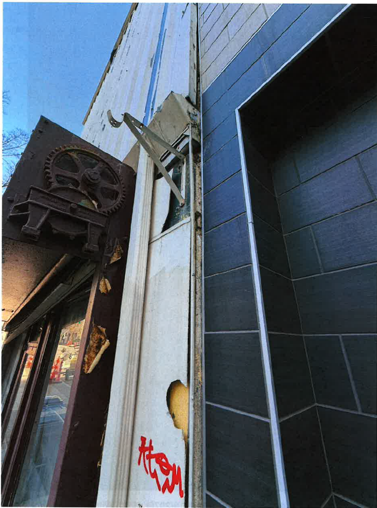
Photo 22: 209 S. Wilmington St Raleigh, NC (03/19/2026) Detail of 209 S. Wilmington St. wall independent of 211 S Wilmington St. Evidence of stucco direct to brick can be seen.
