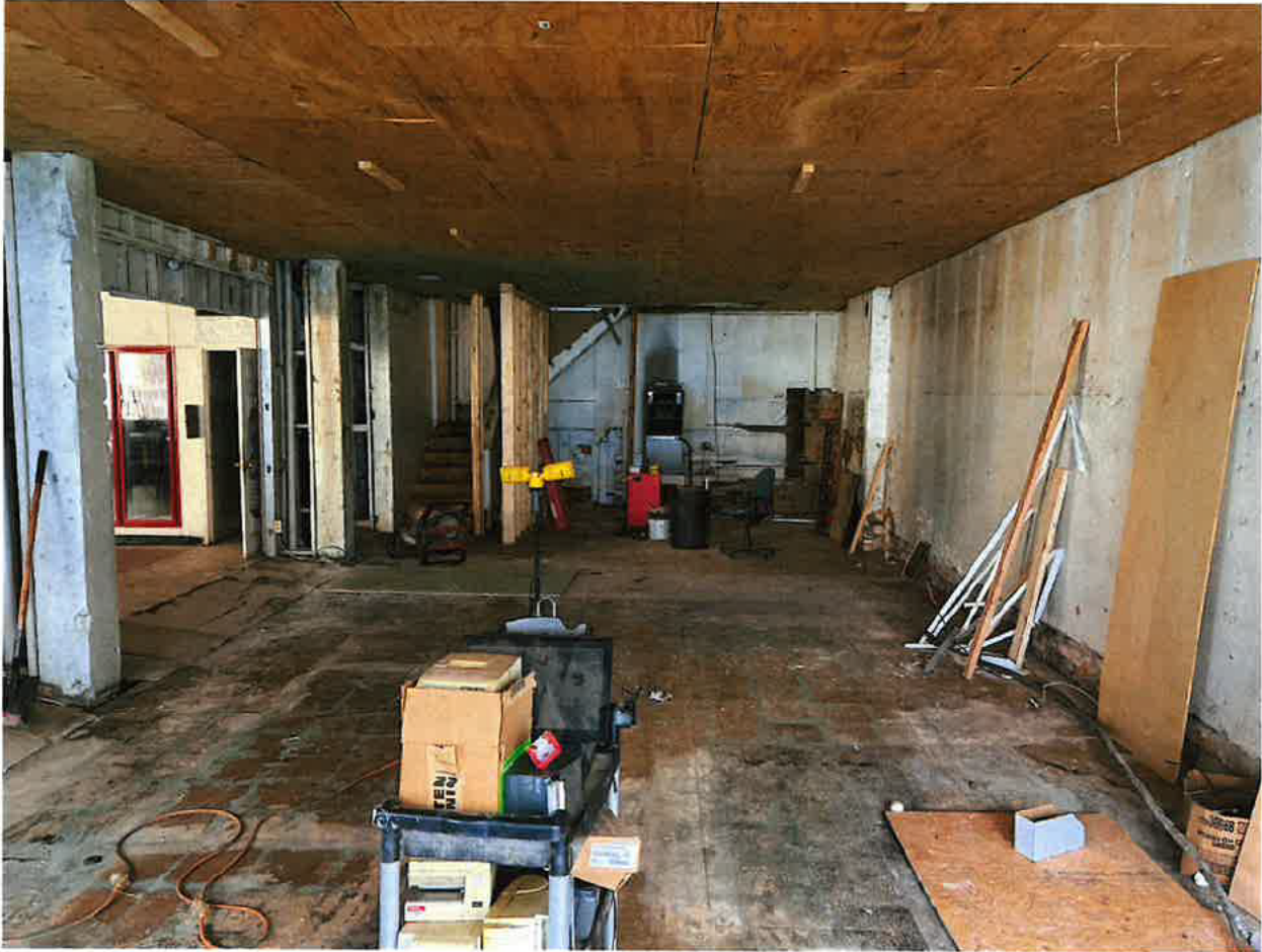
Photo 4: 209 S Wilmington Raleigh, NC (03/19/2026) 1 st floor, Interior Facing East. No original ceiling material remains, all plywood clad in floor joists. Rear stairs are not original and in disrepair.
