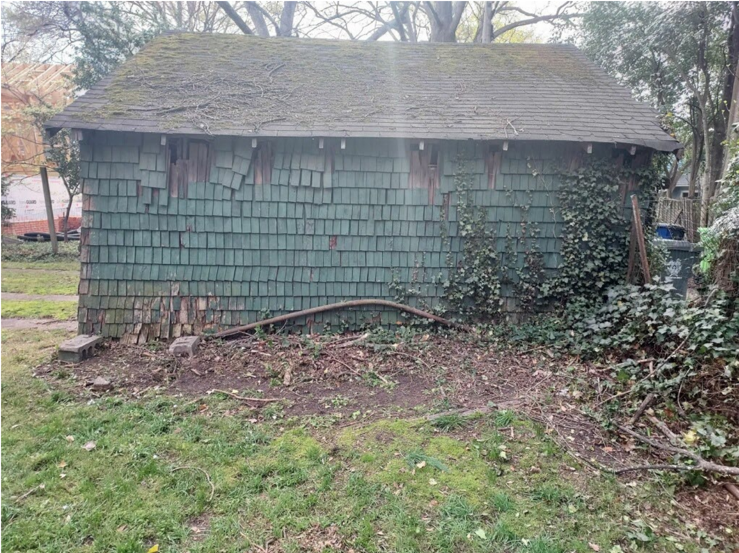
Outside West facing wall of garage, showing deterioration
