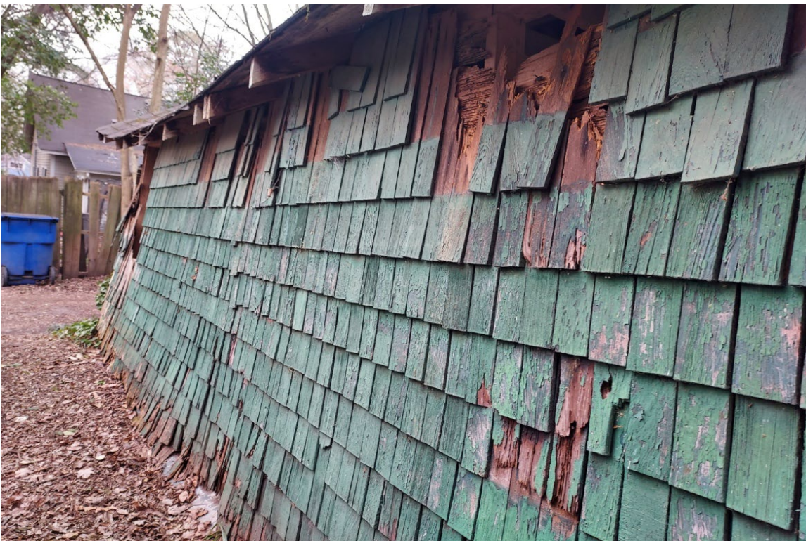
Damage to outside East wall from the front corner of the garage
